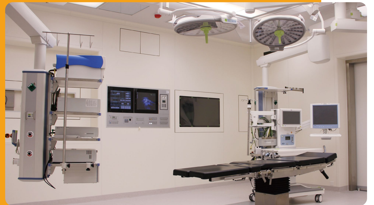
Industrial Touchscreen Display
